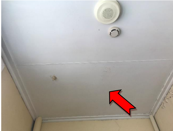
Photo 1. Interior, level 1, male bathroom, ceiling – asbestos-containing fibre cement sheeting.
