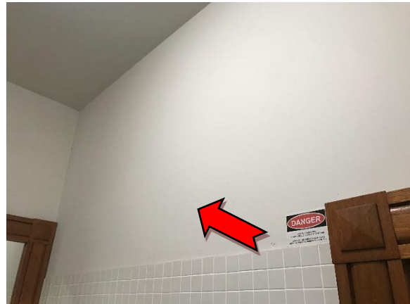
Photo 4. Interior, ground level, male change room – asbestos-containing fibre cement sheeting.
