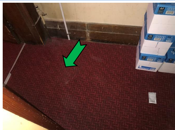
Photo 6. Interior, ground level, western stairs beneath carpet, debris – non asbestos-containing vinyl floor tiles.
