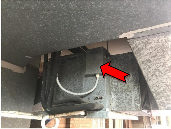
Photo 7. Exterior, western elevation, heater bank – suspected asbestos-containing millboard insulation.
