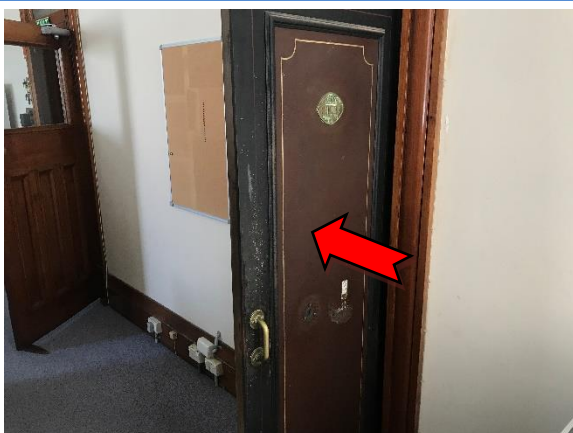
Photo 5. Interior, ground level, strong room, door – suspected asbestos-containing fibre cement sheeting.
