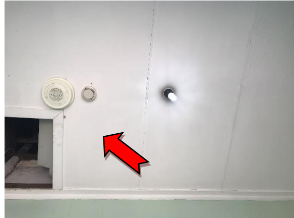
Photo 2. Interior, level 1, female bathroom, ceiling – asbestos-containing fibre cement sheeting.
