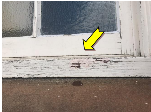
Photo 10. Exterior, throughout, window frames - suspected lead-containing white upper paint system.
