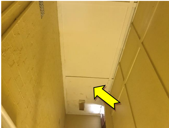
Photo 9. Interior, throughout, ceiling - suspected lead-containing white upper paint system.
